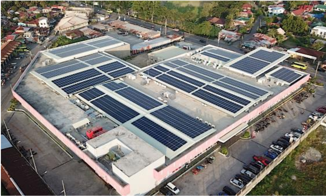
Source: Information provided by Alternergy; SPCC rooftop – CityMall Victorias City, Negros Occidental
